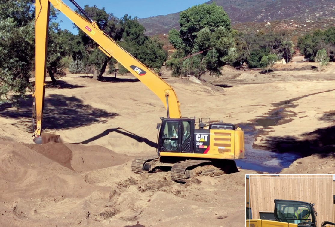
Left: MB General Engineering, Inc. utilizing a Cat 326F long reach excavator from Hawthorne Rentals to perform lake restoration at Point X Camp in Aguanga.
