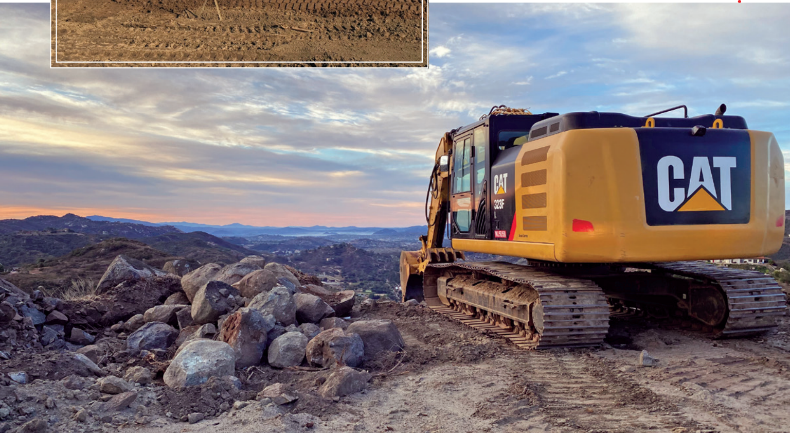
Below: Grading remote house site and pad at Hidden Meadows near Escondido.
