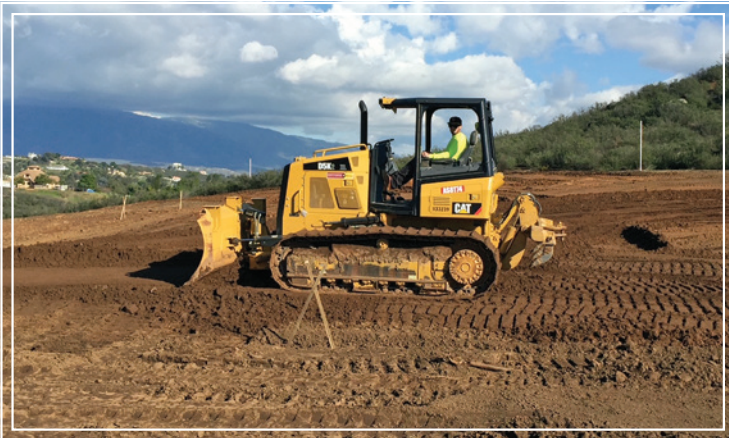
Left: Grading pad for tasting room at Jack Simon Winery in Valley Center.
