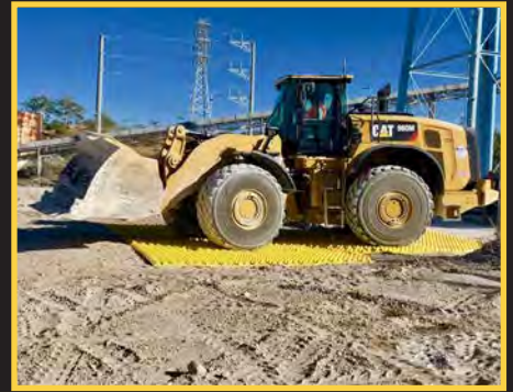
● Industrial Gypsum Plant
